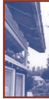
Open eaves, vents not screened (6 pts)
